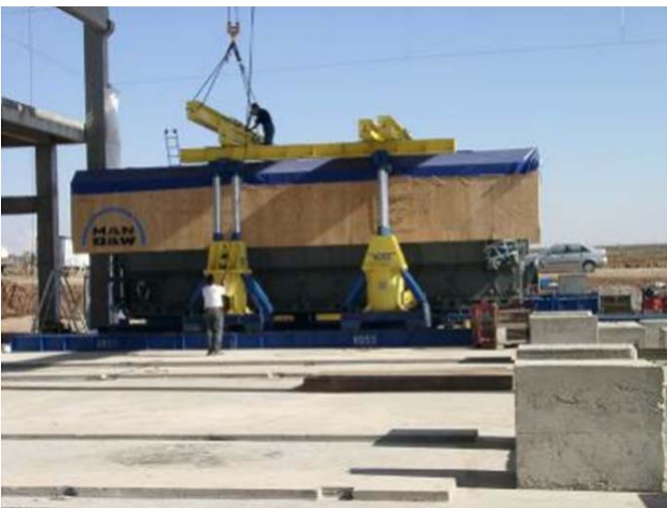
Placing each engine onto the foundation was part of the contract for a total of 6 diesel engines from the production plant in Germany resp. Great Britain to Batman, Turkey
