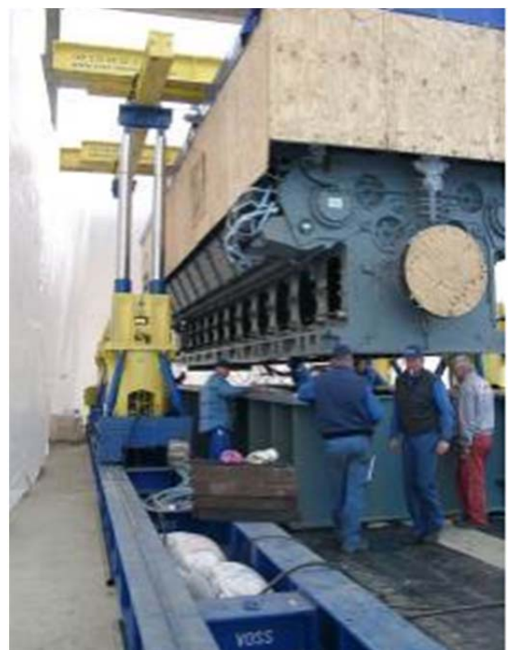
Mounting the engine on the foundation where the oil pan was integrated.
